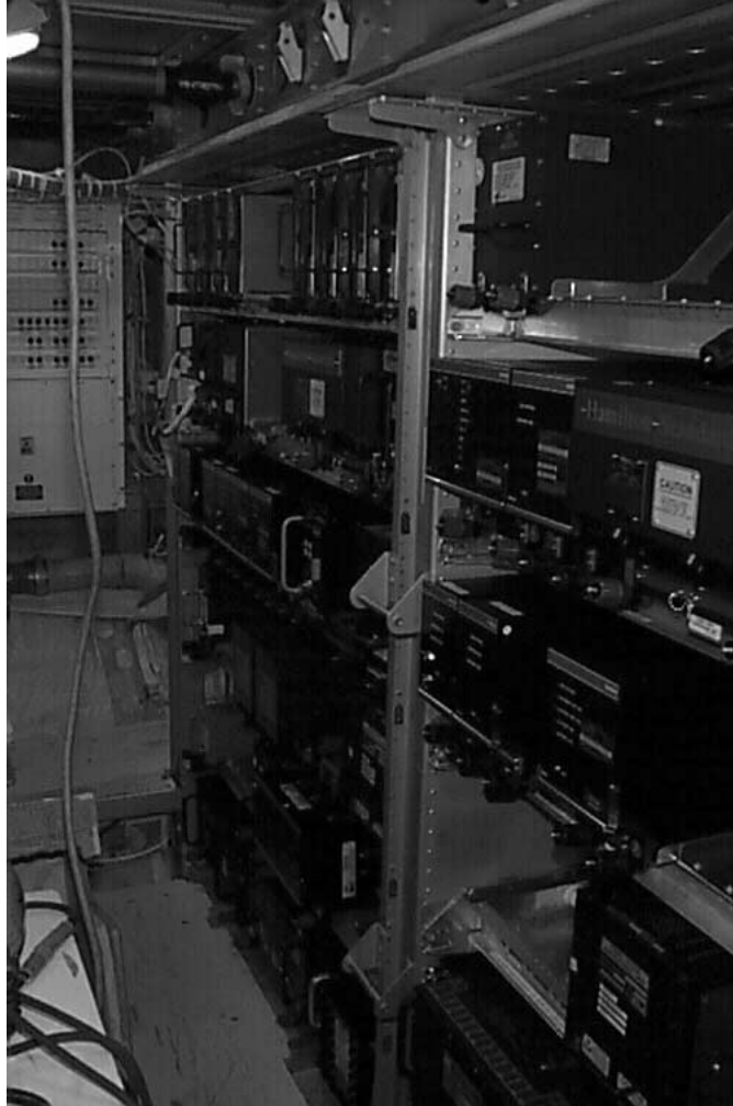
Figure 4.0-16. Typical E/E Bay (2)
