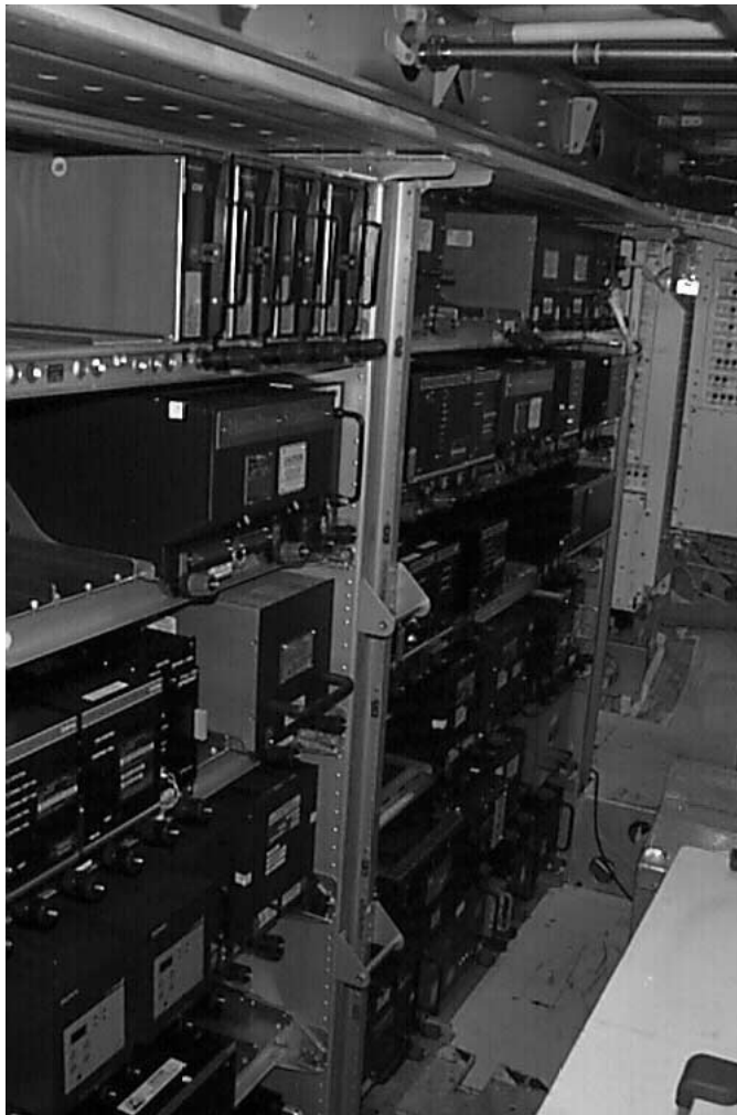
Figure 4.0-15. Typical E/E Bay (1)
