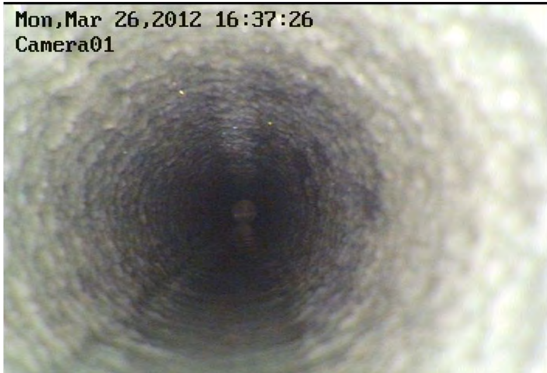
(a) 3/4" Un-Insulated Stainless Steel, Downstream
