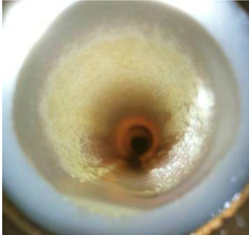
(a) Un-Insulated, Downstream
