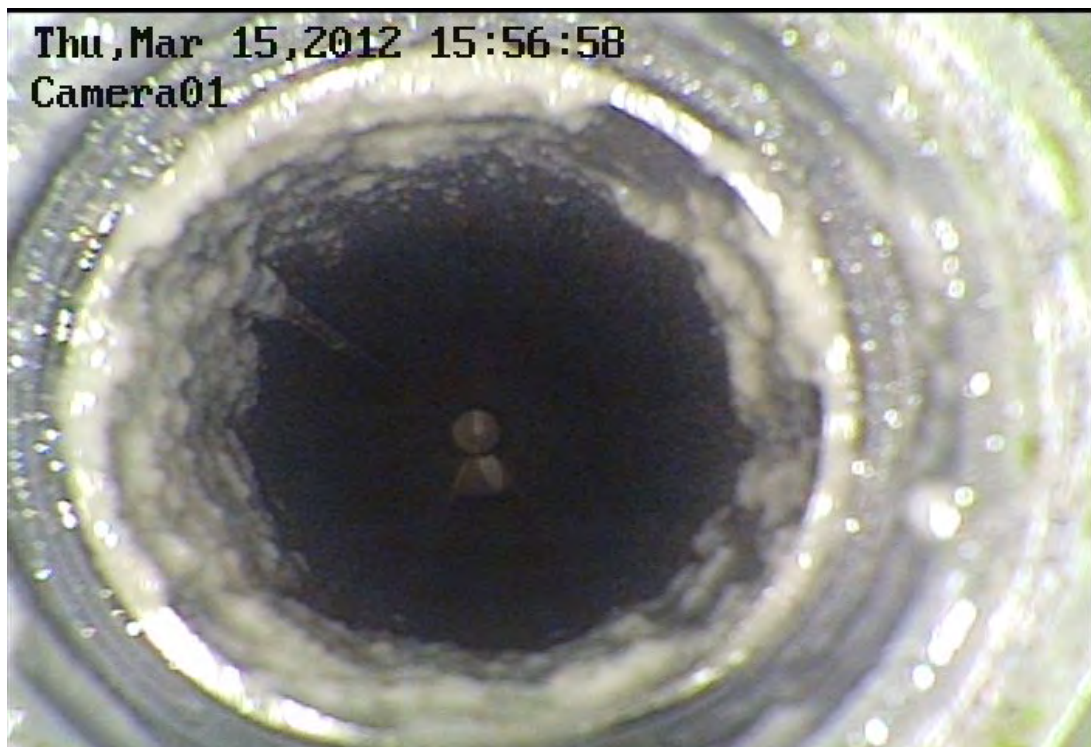
(b) 3/4" Insulated Stainless Steel, Downstream
