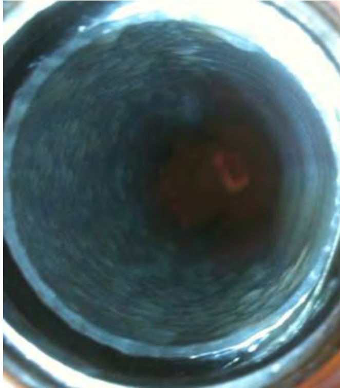
(a) Un-Insulated, Downstream
