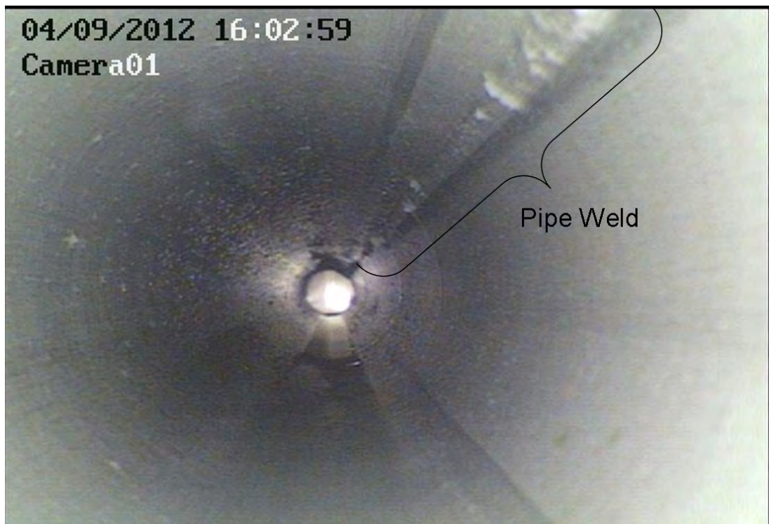
(b) Pipe Oriented right-side-up, T = -11\text{ }^{\circ}\text{C} , Downstream
