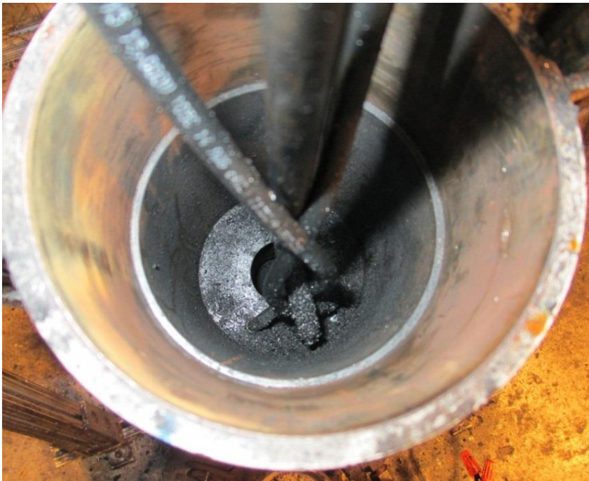
Soot buildup in burner
