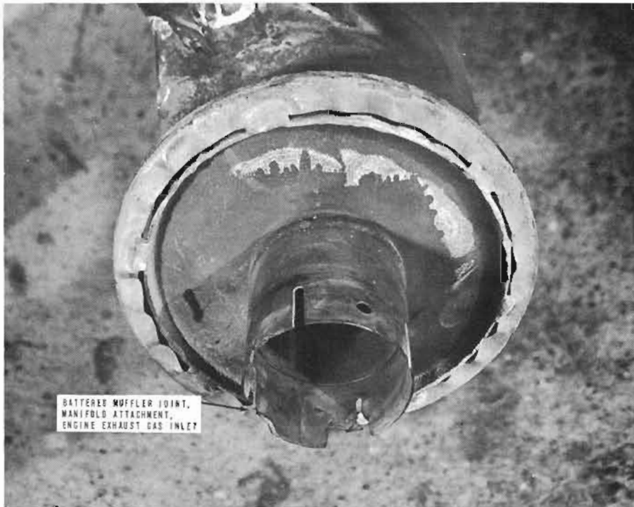
FIG. 1.11 BATTERED MUFFLER AND MANIFOLD JOINT
