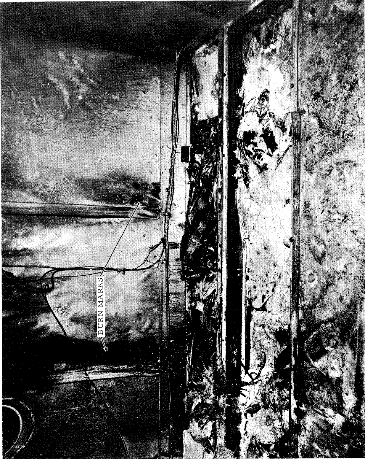
FIGURE 12 - AREA OF FLOOR FIRE
