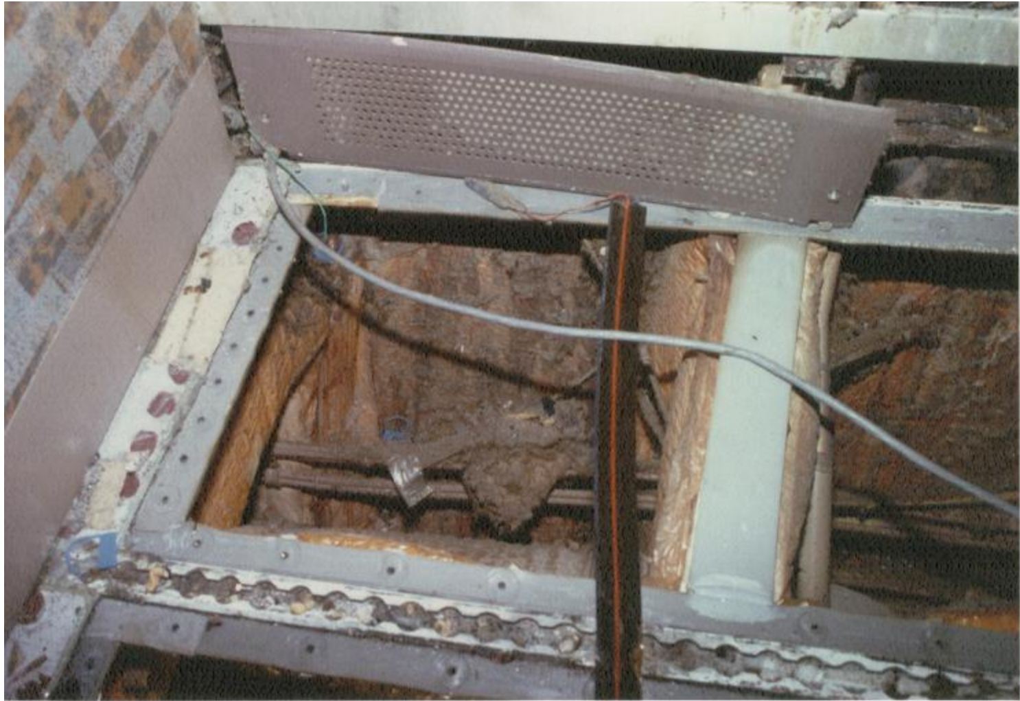
Delta L1011: Electrical fire in check area (Lint and dust on insulation)
