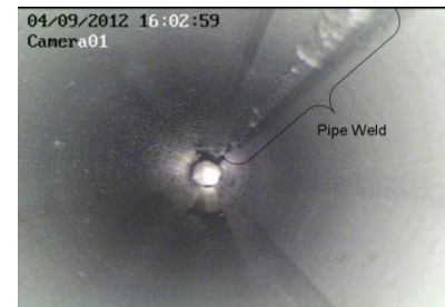
Pipe Oriented right-side-up
